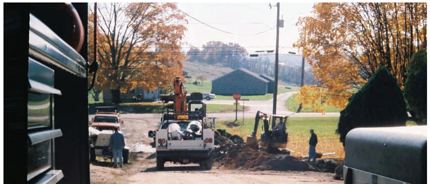
Work begins on upgrading water lines and extending laterals to homes in Ripplemeade, Virginia.
