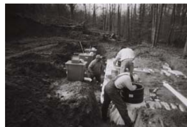
Workers install the rainwater harvesting collection tanks and mixing mechanisms which are buried underground.
