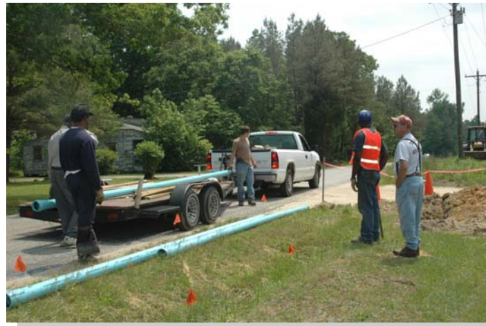
Sections of water line are off-loaded next to the planned pipe route.
