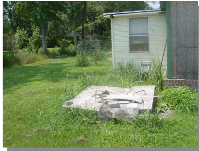
This damaged septic tank cover is an example of the problems plaguing the Annie Village community's overall waste water treatment system.
