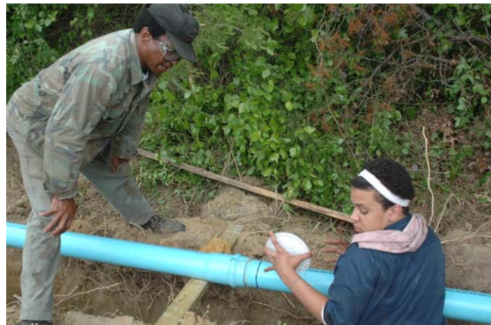
Volunteers glue together sections of pipe. Later pressure testing will insure proper coupling and no leaks.
