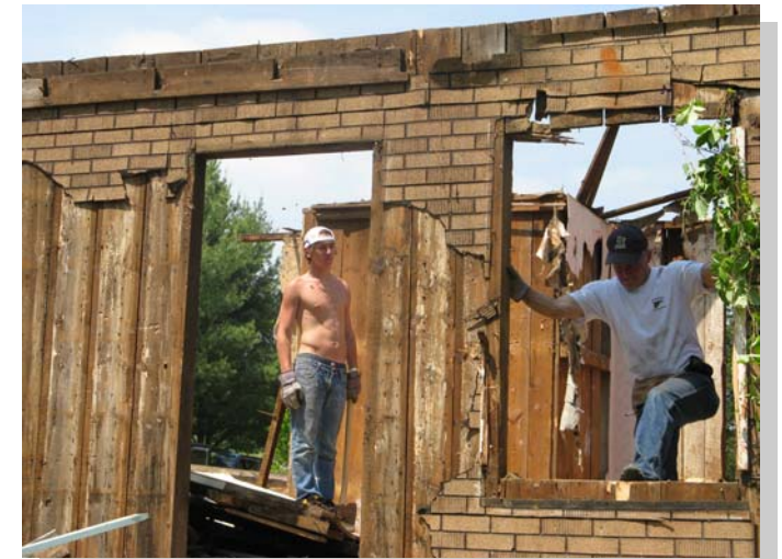
St. Joseph's University volunteers demolish an abandoned house in Barren Springs, Virginia.
