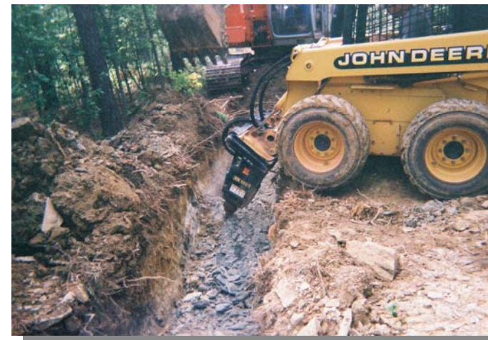
About ten veins of metamorphic rock like this had to be busted out for the 800 ft. of water transmission line from the well to the town's main water line.
