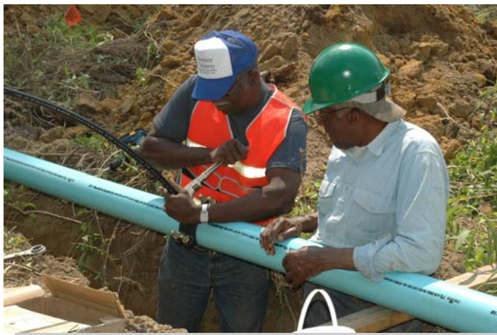
These volunteer workers are tapping the main water line with a one inch connection line which will serve an individual home.
