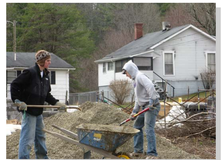
St. Joseph's University volunteers work in Town of Pulaski, Virginia on a Habitat for Humanity project bringing water to a family previously lacking indoor plumbing.
