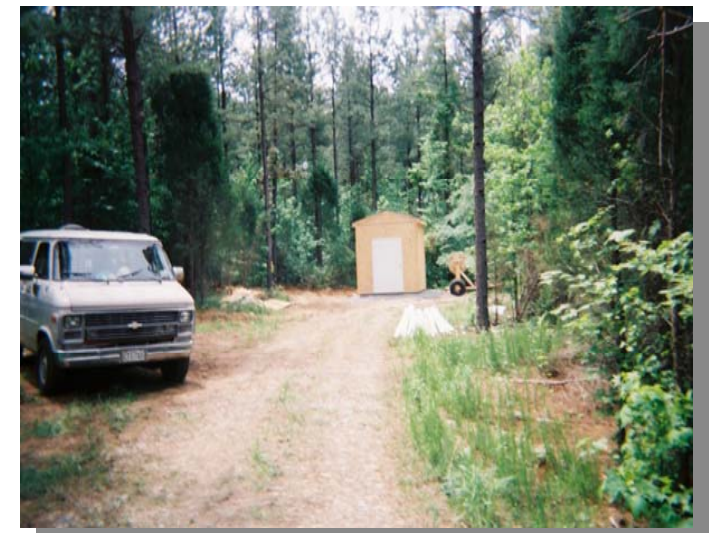
The new well house for pumping and treatment is located on a well lot and access road graciously granted by a Virgilina landowner.
